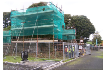
Major conservation works were carried out to save Tulsk priory from collapse
